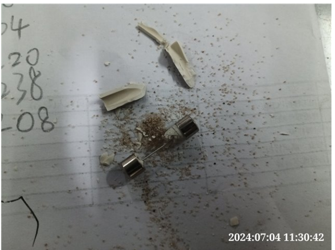
Photo# 214 Fuse check
