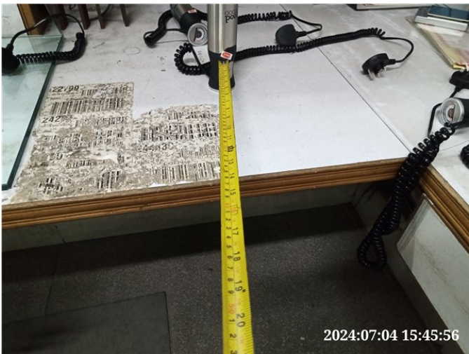
Photo# 13 Poor painting - minor
