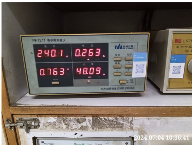
Photo# 97 Power consumption test(motor appliance)
