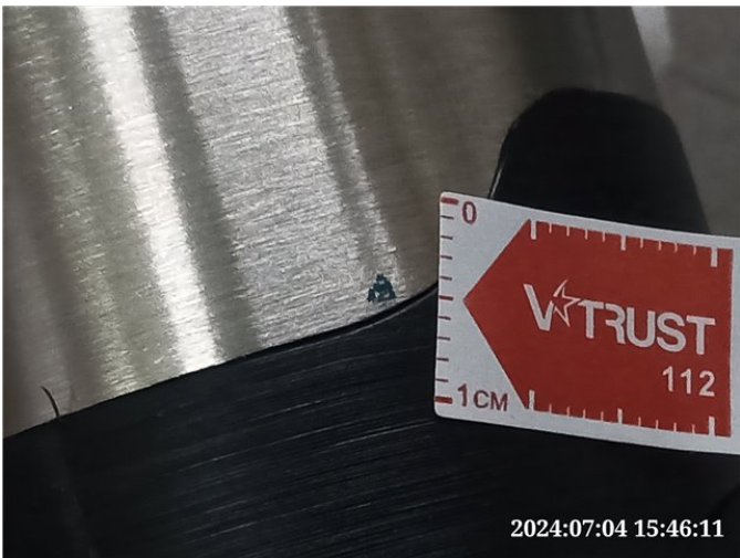
Photo# 14 Poor painting - minor
