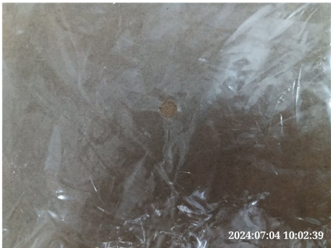
Photo# 186 Air hole
