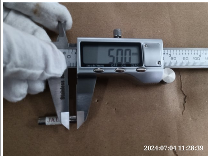
Photo# 213 Fuse check
