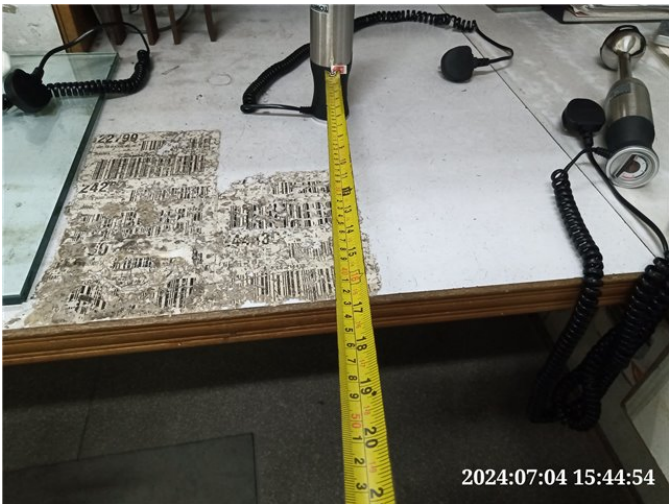
Photo# 11 Poor painting - minor
